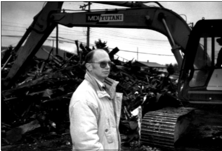
LOST PAPER – Dave Scherger, former publisher of the Spectator in 100 Mile House, B.C., watches his offices being demolished.
