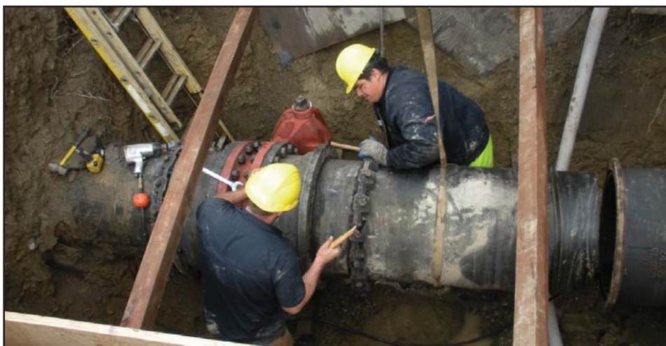
City of Kent Water Department installing 24" butterfly valve on incoming side of their water supply to the valley floor.
