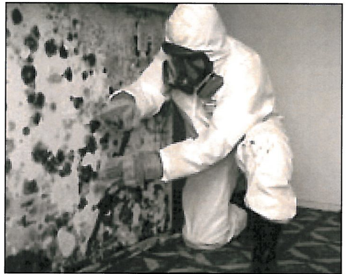
Mold thrives in wet conditions, such as is found following a flood. Here, mold grows on a wall, and a worker is wearing adequate protection for safety. Photo courtesy U.S. Environmental protection Agency.
