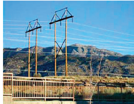
230 kV transmission line. Notice the three wires or conductors hanging from each tower. Three or four wires generally will signify a three phase transmission line.
