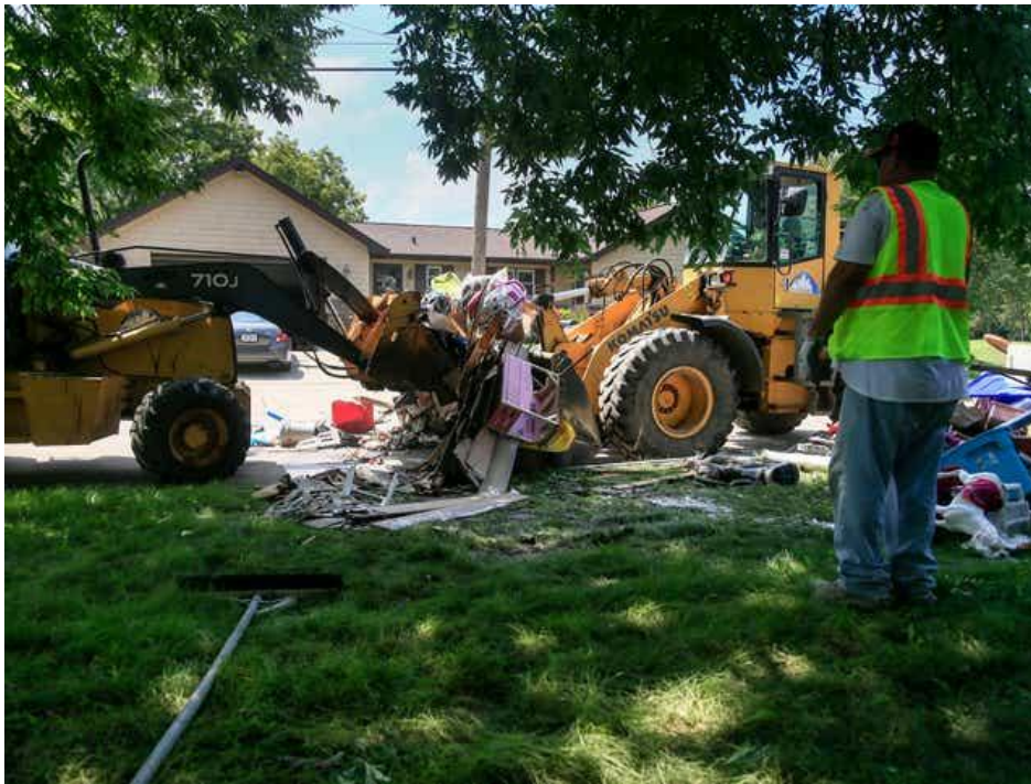
City workers load destroyed belongings from flood-damaged homes on East 35th Street in Des Moines on Tuesday, July 3, 2018.
