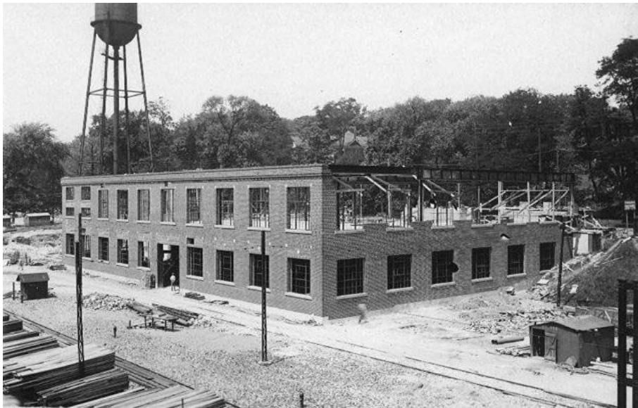
Davenport Garage under construction, looking northwest, July 6, 1925. Photo by Alfred Pearson. City of Toronto Archives, Fonds 16, Series 71, Item 3888.
