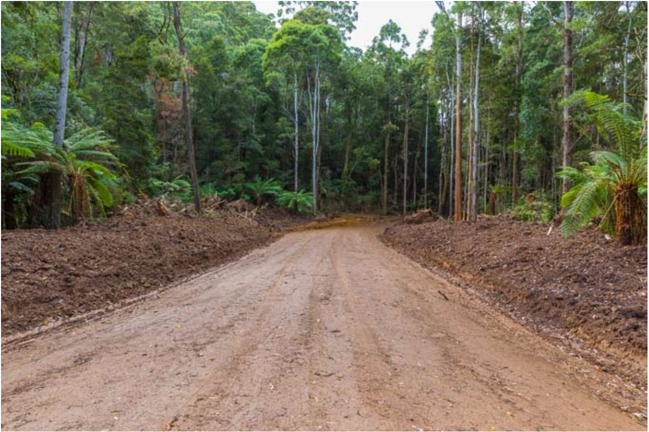
Above: Evidence of new roading, taken 2/2/2017.
