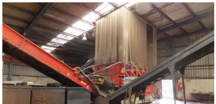
Shredder – fitting these screens at TIC has suppressed most dust operation and restricts pollution escaping the site.
