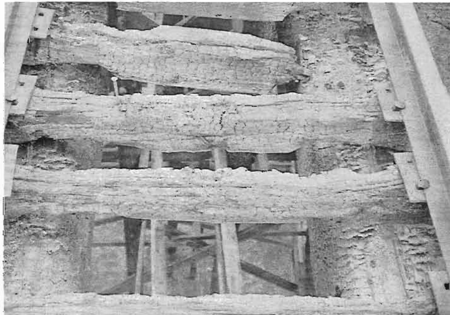
This closeup shows charred ties, one of which is burnt through. Photo by G. Frederick Stork
