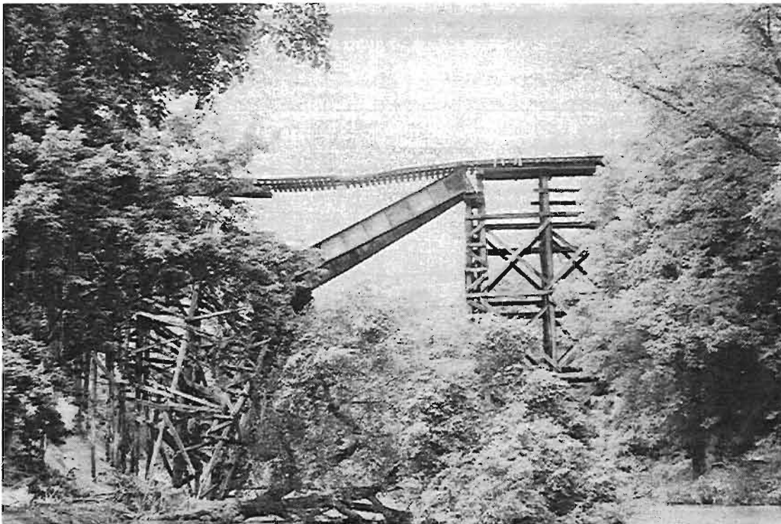
The sad condition of the battered bridge after Agnes in 1972. The shattered support structure on the left (the west) was removed and steel supports were built.
