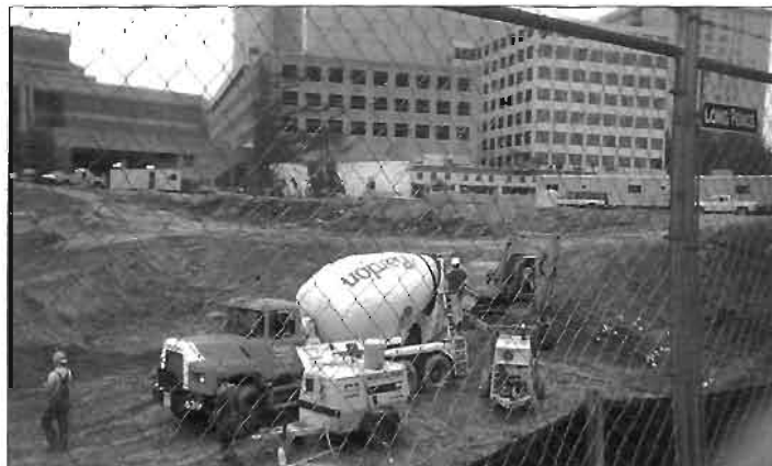
Federal Realty Investment Trust broke ground last summer on its "Phase IV" Bethesda Row development at Bethesda and Woodmont Avenues, adjacent to the CCT/Wisconsin Avenue tunnel (upper left, behind the trailer). Plans call for 25,000 square feet of street retail, 80,000 square feet office space, all of which will be located above a 35,000 square foot subterranean art screen cinema. Completion date is scheduled for Fall 2000.
