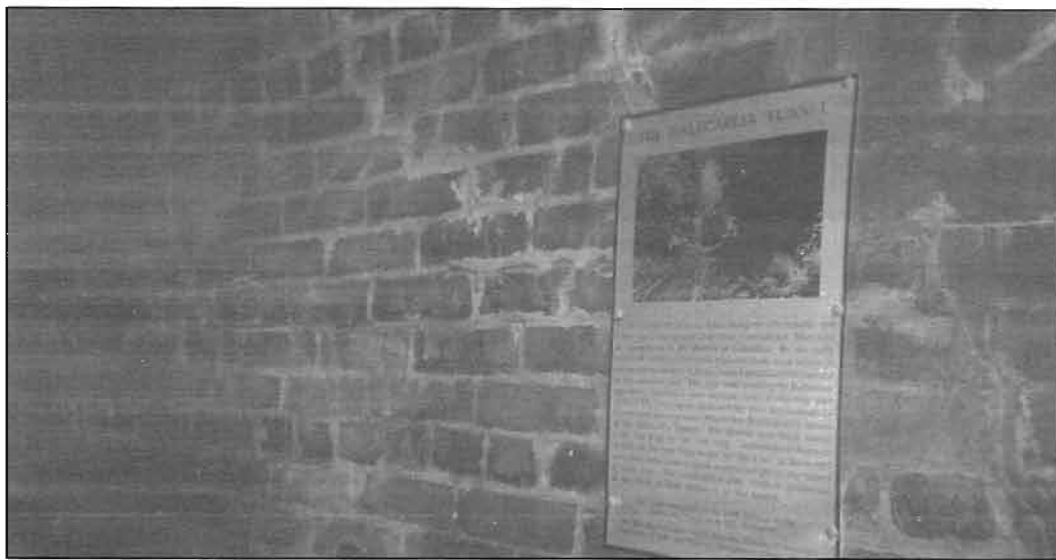
Last summer, Montgomery County Parks coordinated graffiti removal operations at the Dalecarlia Tunnel. The CCCT met with Parks officials to discuss the best way to remove graffiti. Power washing was rejected as being potentially too damaging to the old mortar joints, so crews did their best with wire brushing. Other approaches to removing graffiti are being researched.
