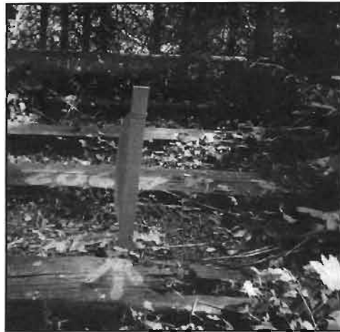
Survey stake marks the start of the construction phase for the Rock Creek trestle.
