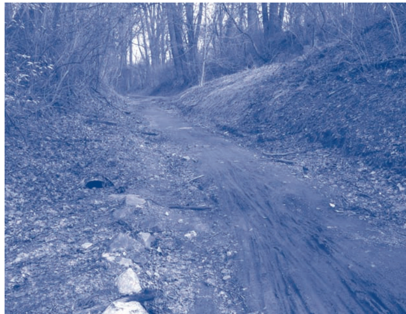
The crushed stone trail surface has completely washed away near the Silver Spring end. An approximate half mile section of the trail badly needs repair.
