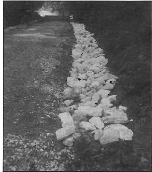
Erosion prevention work along the Georgetown Branch/ Capital Crescent Trail near the 0.5-mile marker.
