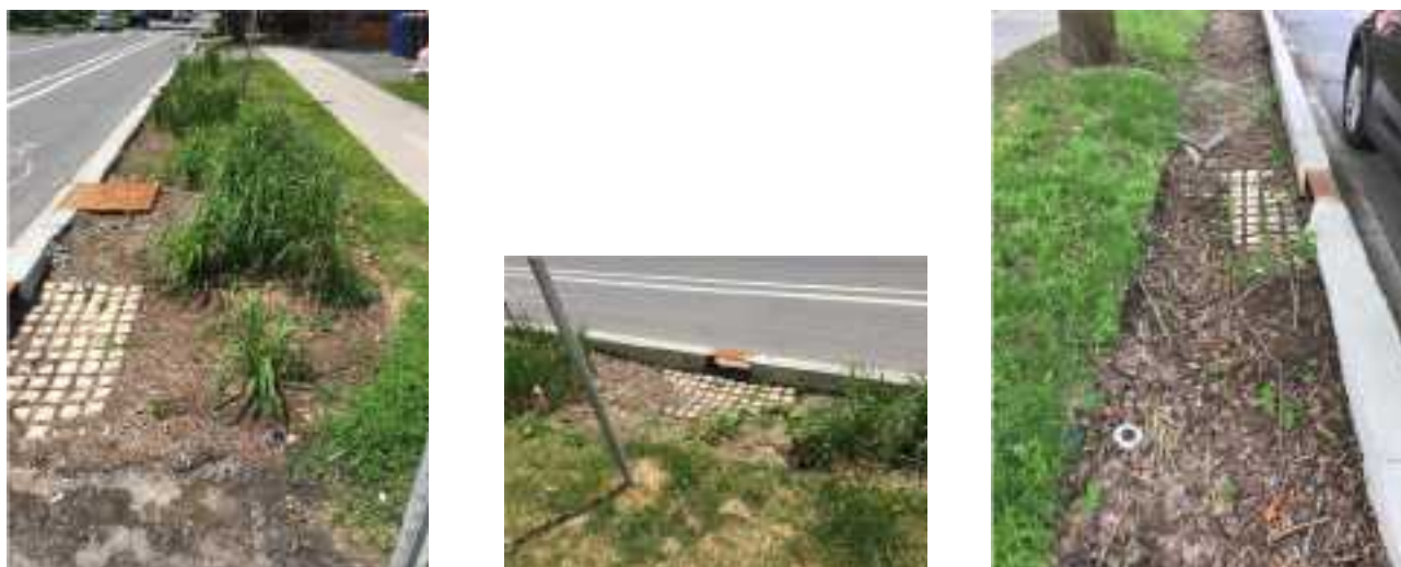
FIGURE 11: – PHOTOS OF STEWART STREET BIORETENTION PILOT
