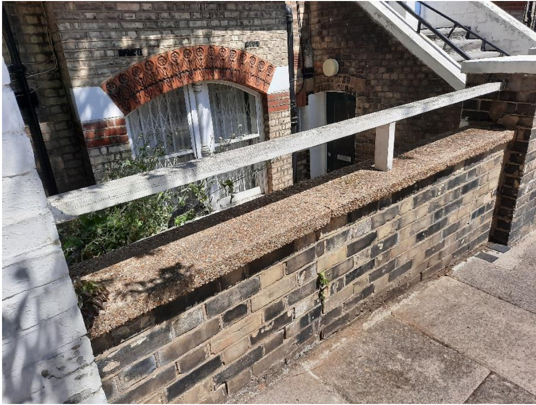
Lengths of 4x2's form make-shift railing in the front, unattractive coping material
