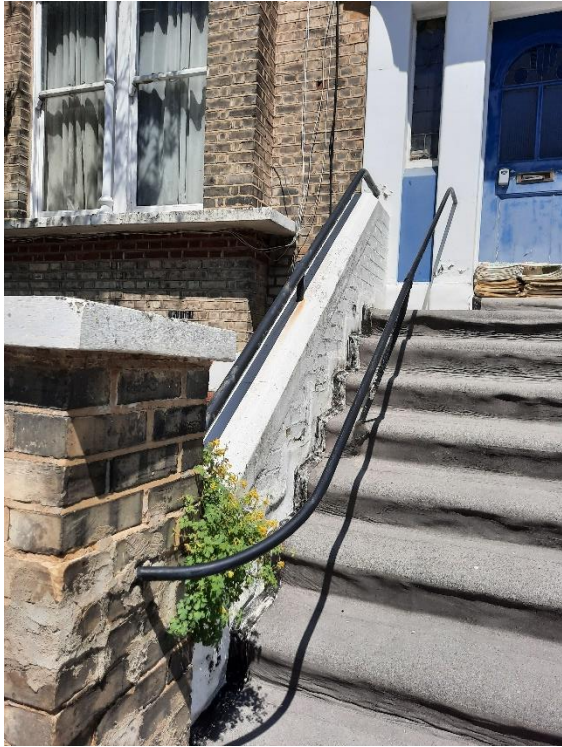
Hand railings at front fail to enhance the entrance; the broad steps are a prominent feature of the building
