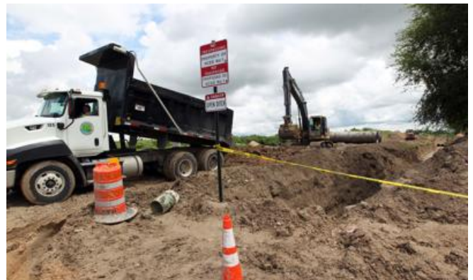
Hidalgo County Drainage District number one workers remove mud from a ditch being built on Rooth Road to connect to another ditch on Saturday, Sept. 15, 2018, in Edinburg. Delcia Lopez | dlopez@themonitor.com
