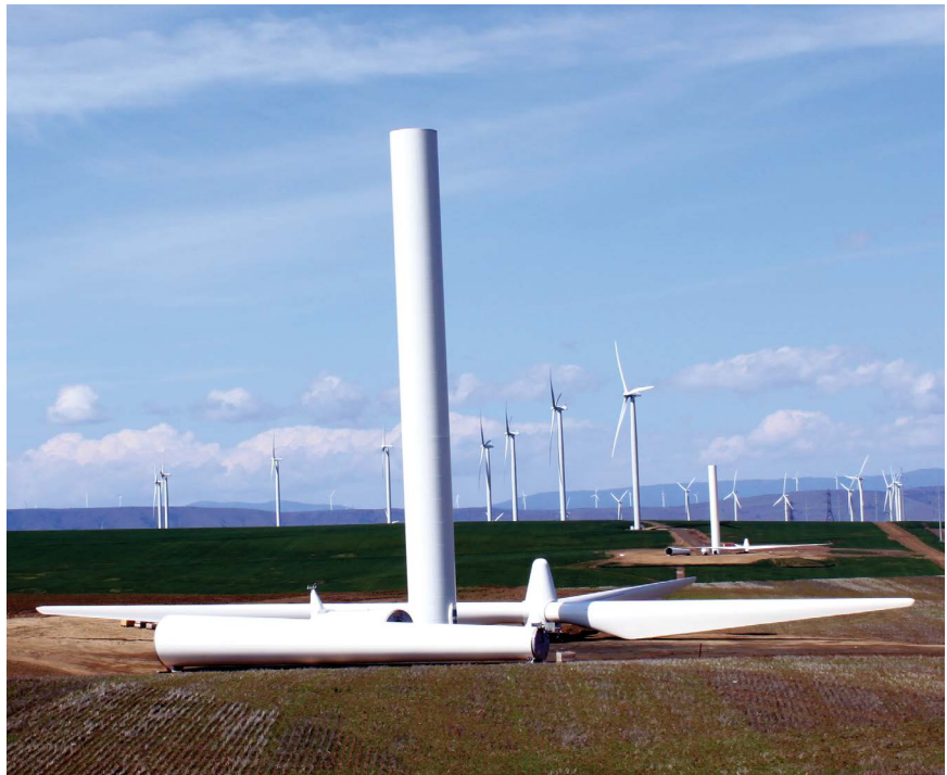
Wind turbines under construction in the Biglow Canyon Wind Farm. Credit: Tedder, cc-by-3.0
