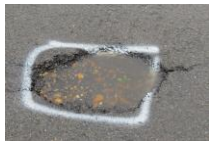
Too many potholes
