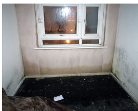
Soaked walls and floor, May Ct
