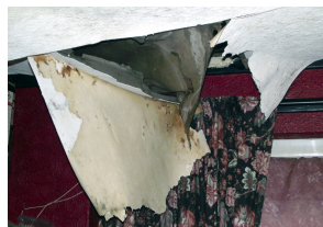
Collapsed ceiling, Birmies
