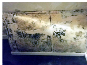
Damp and mould, Gunnet Ct.
