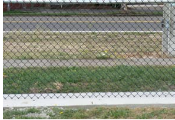
A concrete mow strip under a fence along a sports field in Ida Patterson Park in Eugene.
