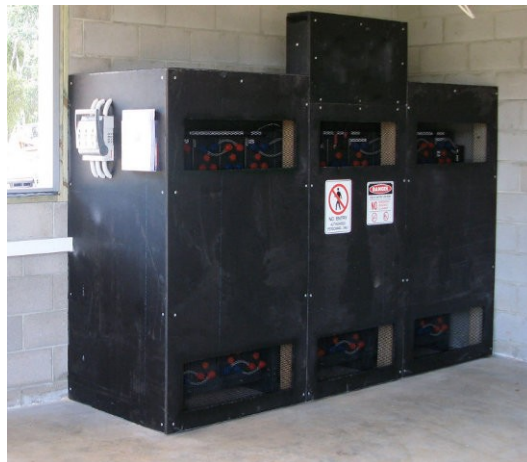
Figure 4: Large battery installation installed to the standards (SolarQuip)
