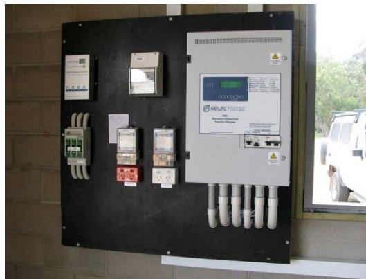
Figure 7: SPS equipment installed to the standards (SolarQuip)
