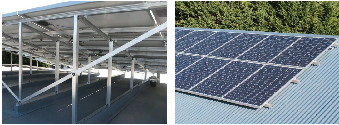
Figure 12: Wind rated solar PV array frames (Elemental Energy, Powersmart)
