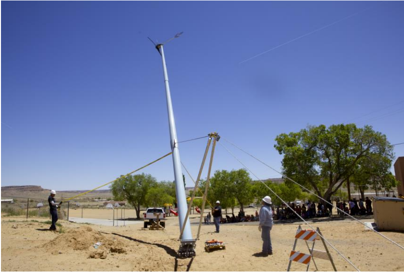
Figure 1. Employees of WestWind Solar and the Hopi Tribe raise a 1.8-kW wind turbine at the Hopi Day School, June 2014. Credit: Daniel Snyder
